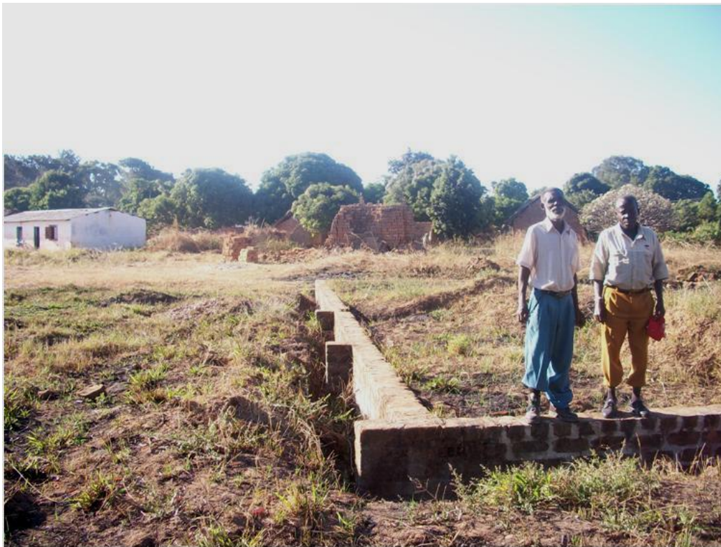
Chair Matthews Mufwaya and Elder Bartholomew Kapeta standing on foundation of church building in progress. Brick kiln made by members in the background and classroom that they are temporarily meeting is far left.
