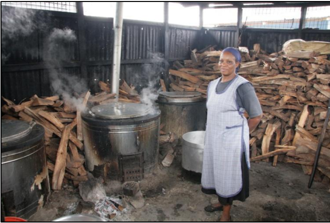
New eco stoves with chimney vents
